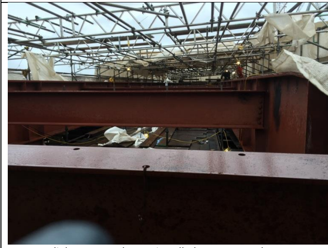
New linkspan cross beams installed- note storm damage to encapsulation
