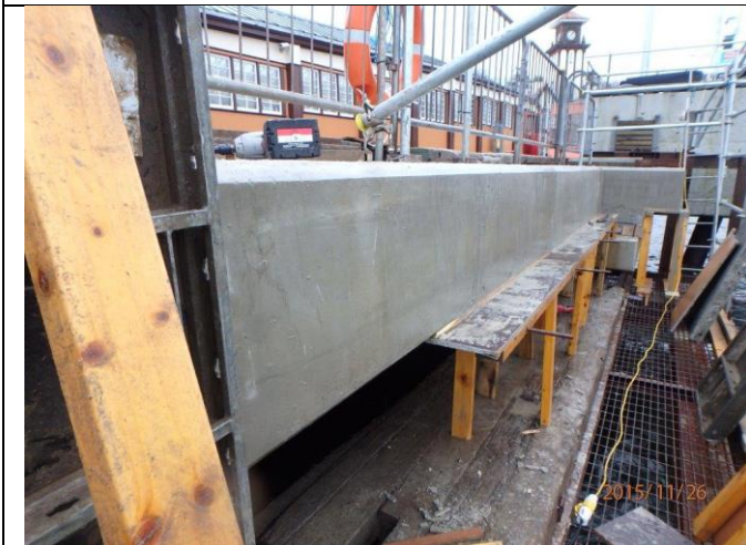
New pier edge after reinstatement. 900mm "notch" along length provides space for new fender system
