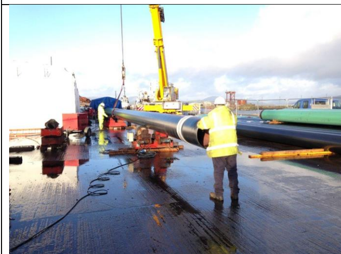
Welding of steel bearing piles at Inchgreen for new roundhead- transported to Wemyss Bay by barge
